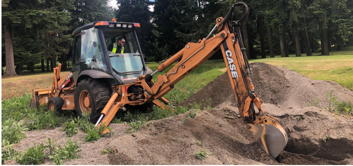
Field Supervisor Tobie Stevens digs a test pit at Cochrane Memorial Park that will guide future design of the park.
